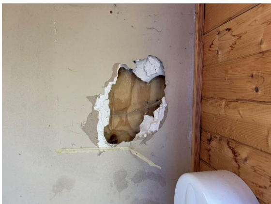
A large hole in the wall - Aha !
